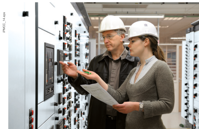
Motor Control Centre (MCC)
